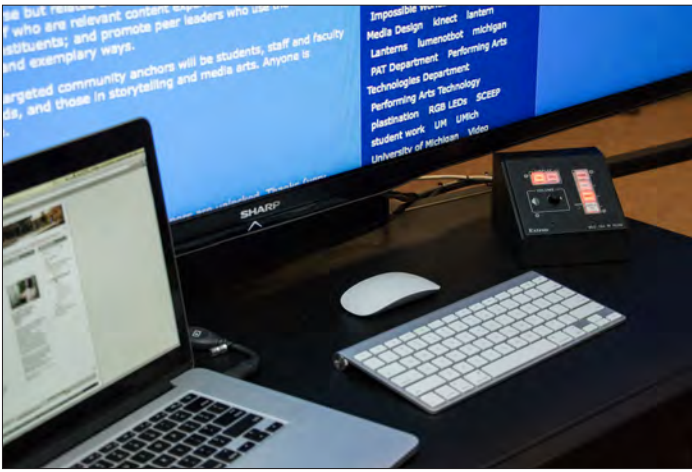
DC Multimedia Rooms Presentation Station- IMG_6019
