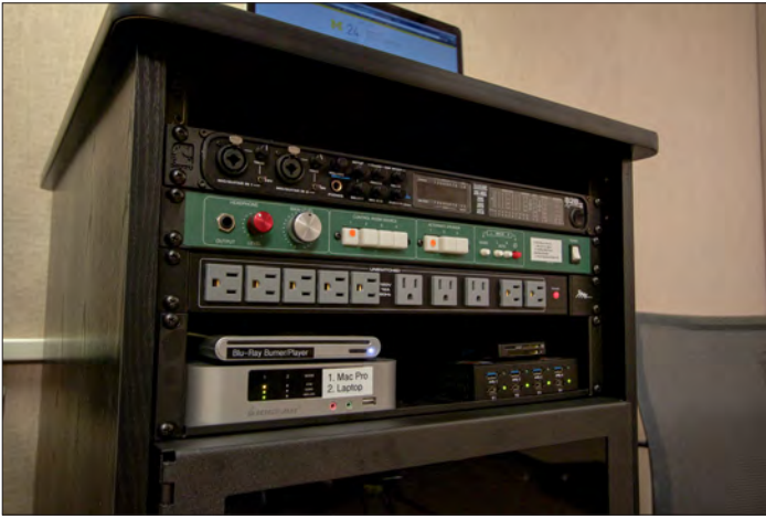
DC Multimedia Rooms IMG_7638
