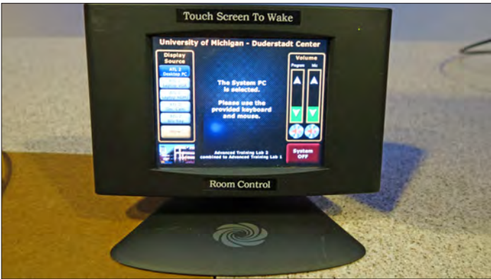
DC Multimedia Rooms DSC00024
