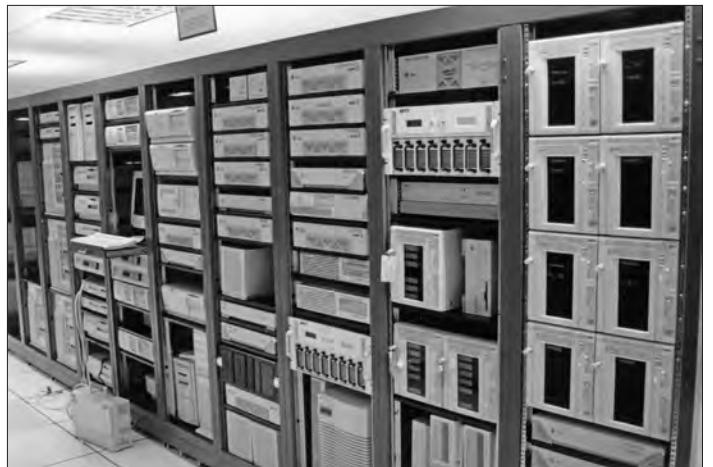
1999MachineRoom Media Union Machine Room
